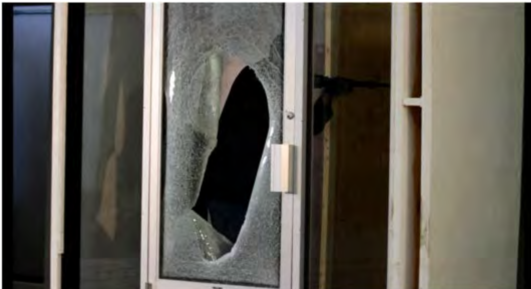
Test #5: Semi-automatic rifle, 3M Safety S140 (14-mil Security Film). Access after 4 gun shots, 11 upper body attacks, 42 kicking attempts, 24 impacts with 9-lb steel pipe. Total time elapsed was 106 seconds.
